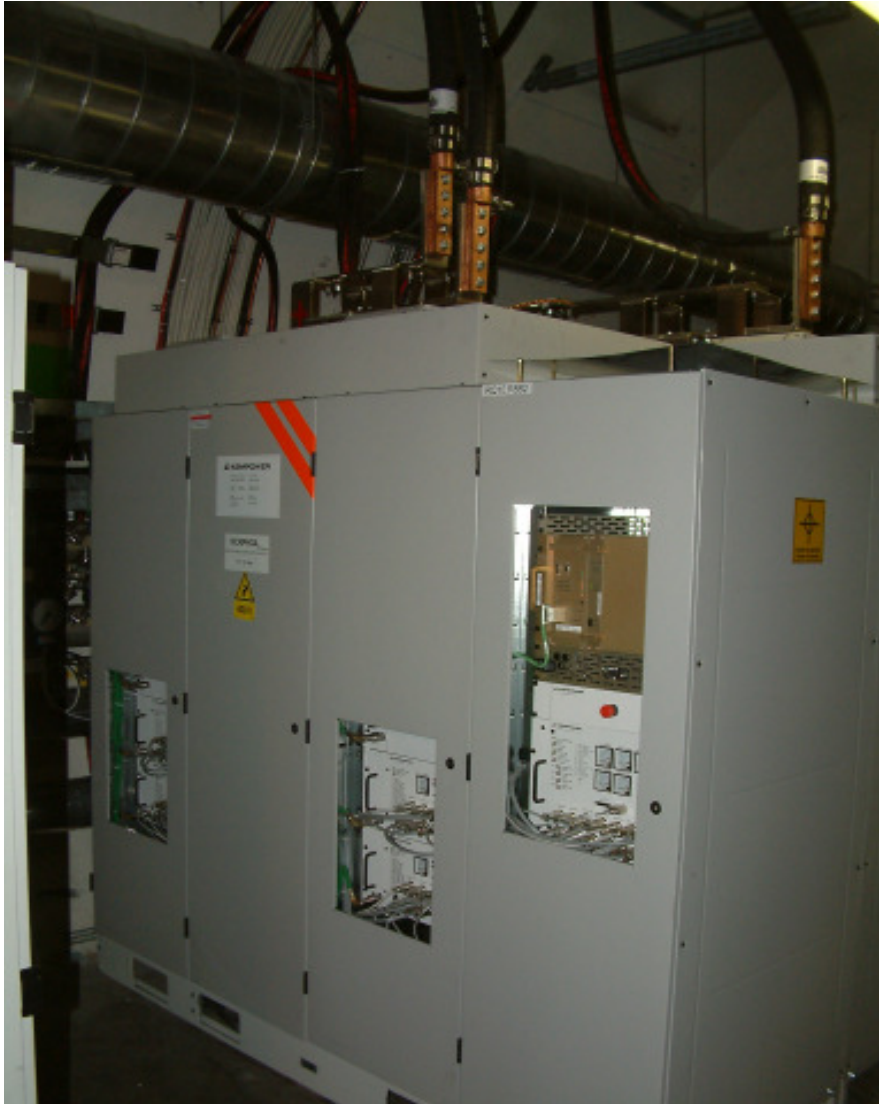
Power converter 6 kA
