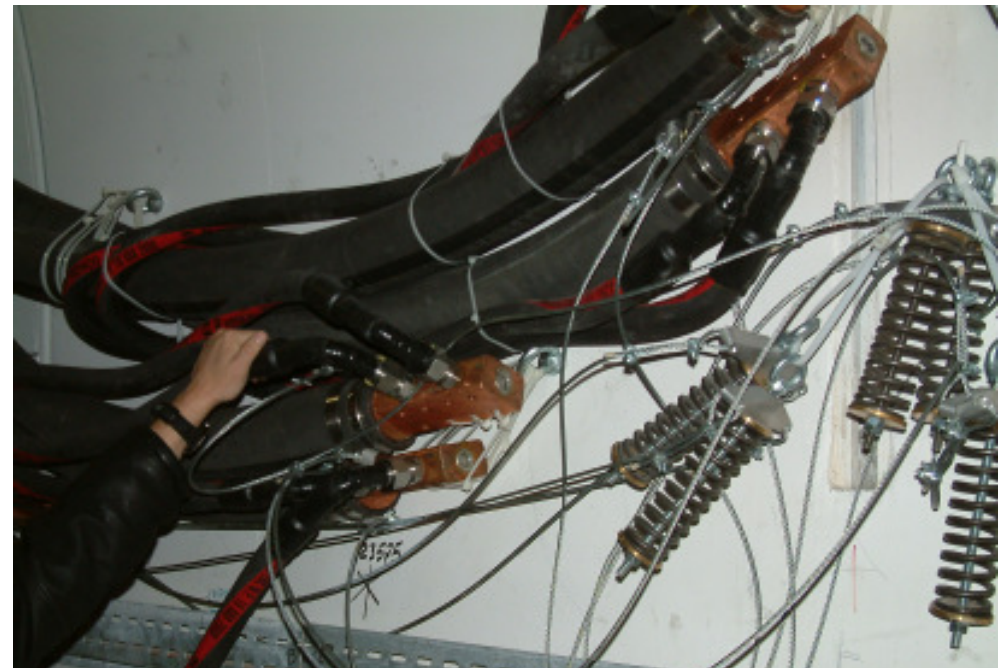
Water cooled cables 13 kA
