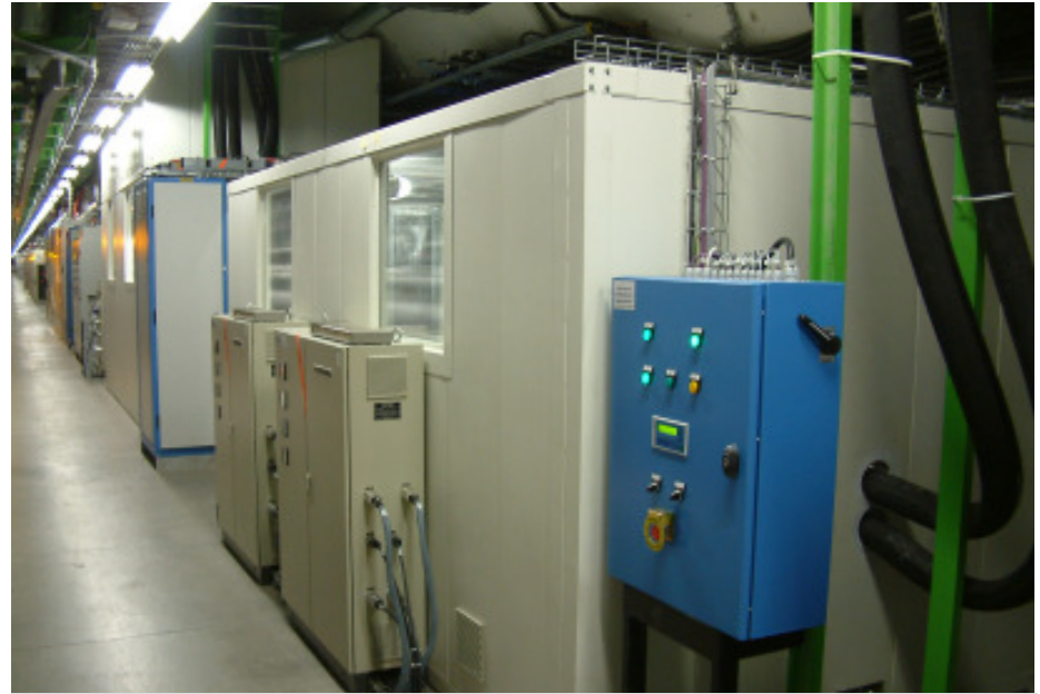
Energy extraction switch house 13 kA
